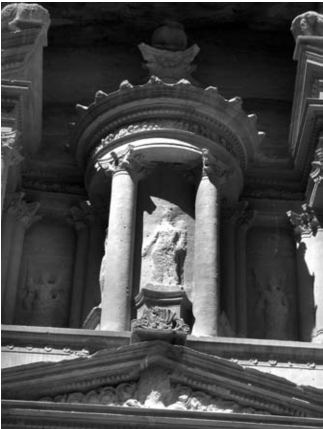
III. 5.30. The tholos crowned by a Corinthian capital and frieze on the facade of al-Khazne at Petra. (Photo: O. Peleg-Barkat)
